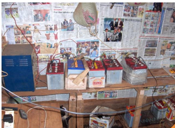
Figure 2. Battery-charging station using old car batteries at the Tungu Kabiri mini-grid in Kenya.
