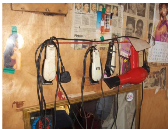
Figure 3. Equipment at a hair salon on the Tungu Kabiri mini-grid in Kenya.
