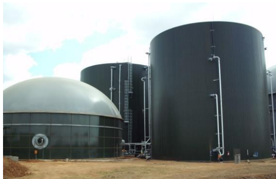
Figure 3. Commercial anaerobic digester using cow manure and industrial waste. Source: Bio2Watt Bronkhorstspuit plant South Africa.
